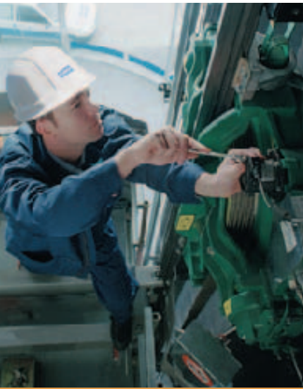
Regular maintenance and the modernization of aging equipment to meet contemporary requirements ensure the reliable operation of elevators, escalators and building doors.
