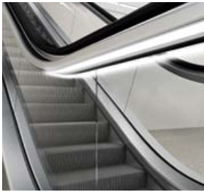
Continuous LED handrail lighting *
