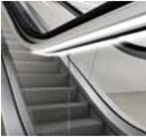
Continuous LED handrail lighting
