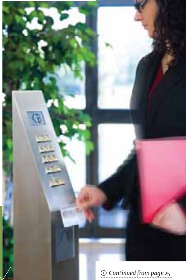
This Schindler ID console serves as an access control system for the building’s elevator bank.
