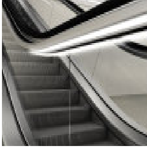
Continuous LED handrail lighting
