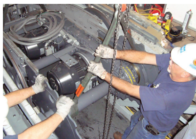
Foreman Danny Richardson and his crew lower the upper EcoMod™ Module into the truss
